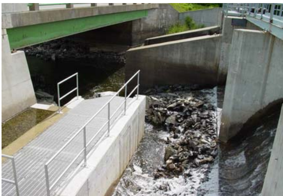
View of the new fishway and viewing platform at the Sebasticook Lake Dam outlet
